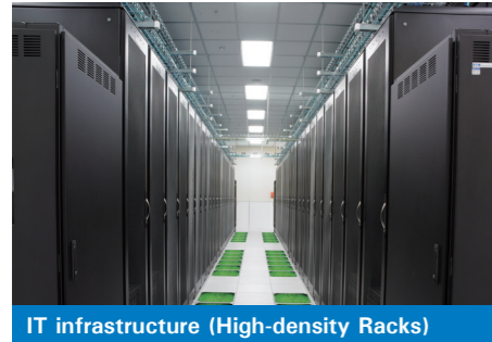
IT infrastructure (High-density Racks)
